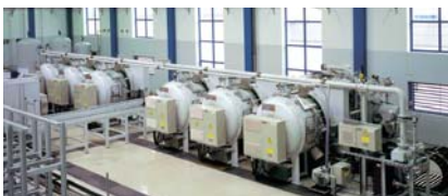
Fig. 6. Production can continue even through routine and many unscheduled maintenance operations.
